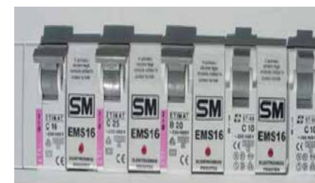
Samodejno stikalo EMS 16 – primer namestitve v el. omarico / EMS 16 demand switch – el. distribution board installation example.
